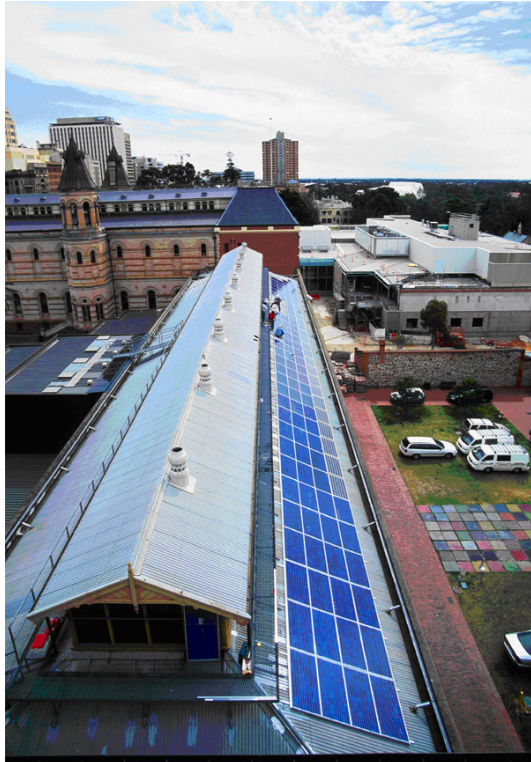
Photovoltaic installation on the South Australian museum
